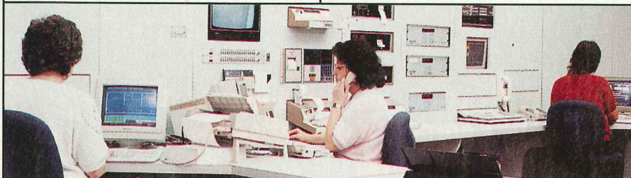
Corporate Protection Services, No. 97, operates a UL/FM-listed central station in Toledo, OH. Photo: Corporate Protection Services
